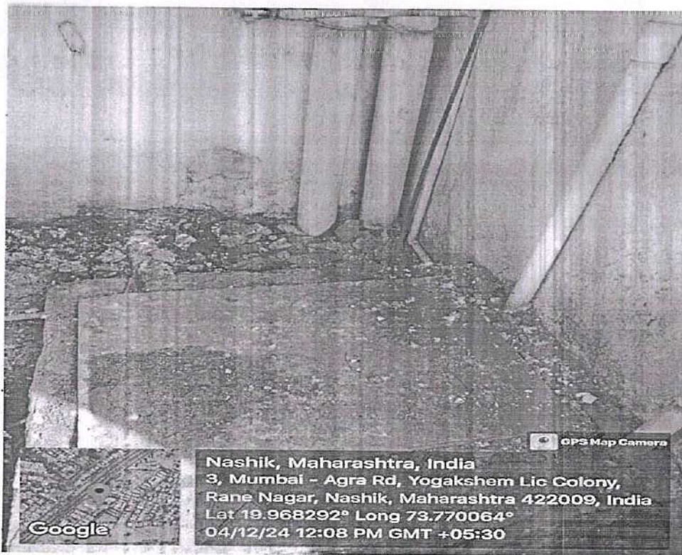
Liquid waste drainage
